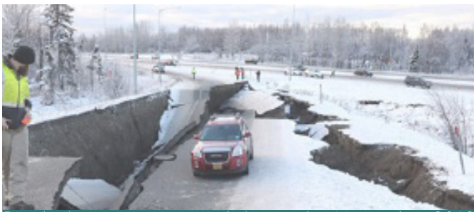
Road damages sustained during the November 2018 magnitude 7.1 Alaska Earthquake 📷 NBC News
